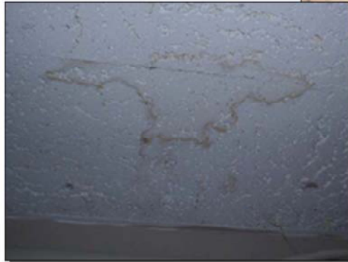
Rodent urine stain in drop ceiling
